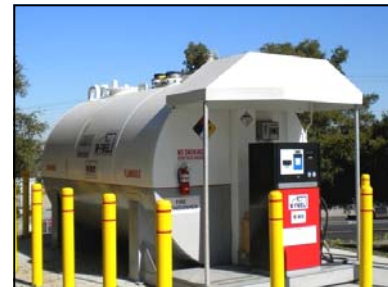
Portable Fueling with Interface to Automatic Tank Gauge
