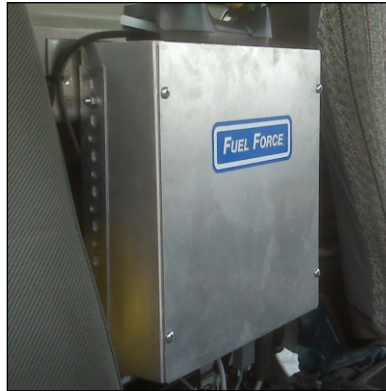
Site Control Processor
